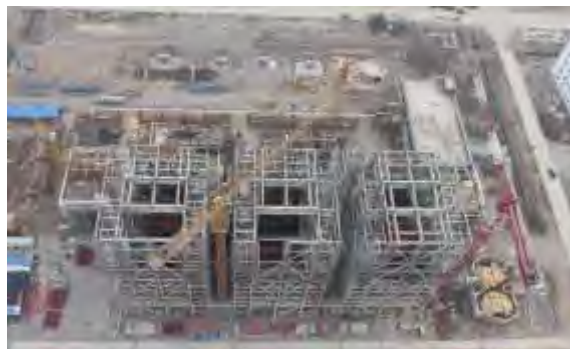
Cogeneration Power Plant in Wuhan Ethylene Project
