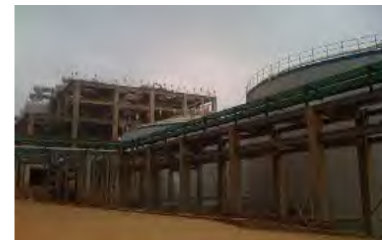
Yunnan Hongxiang Sulphuric Acid & Phosphoric Acid Project
